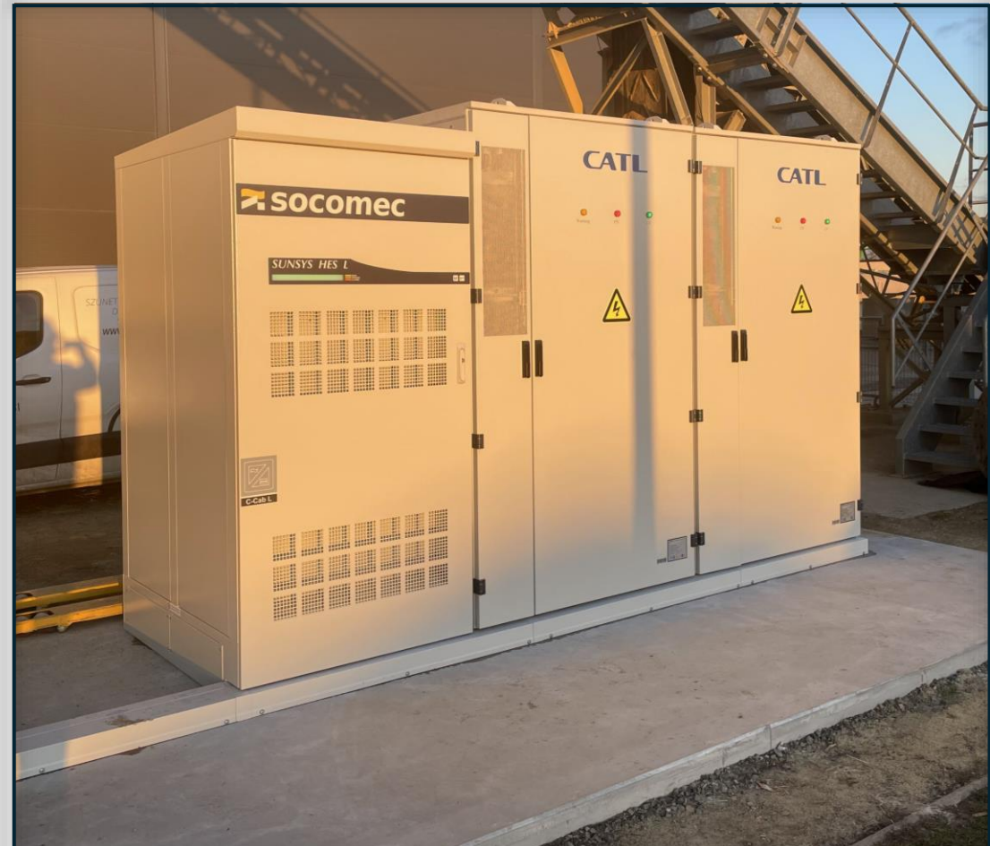
200kW/372kWh Prebeton - Erdőtelek
